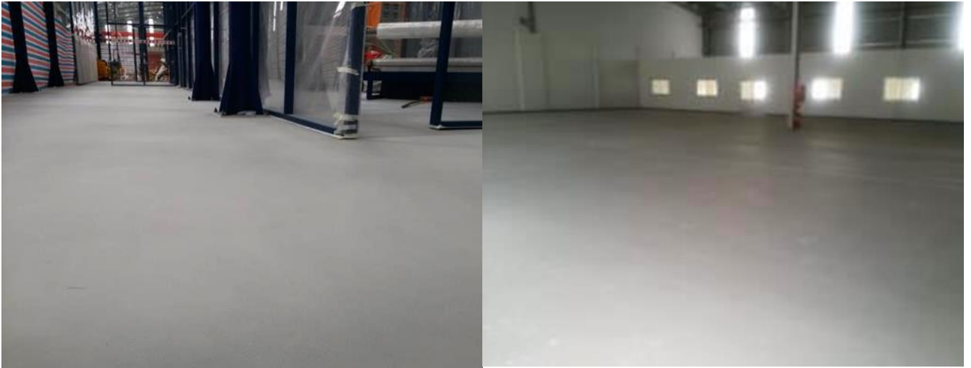
Picture: SikaFloor®-81 EpoCem® New HC was applied at Mercedes factory with system of SikaFloor®-81 EpoCem New HC, SikaFloor®-161 HC and SikaFloor®-263 SL HC
