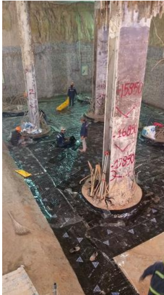
Picture: SikaBit® W-15 was applied at basement of (-18) meters depth in Majestic Hotel project
