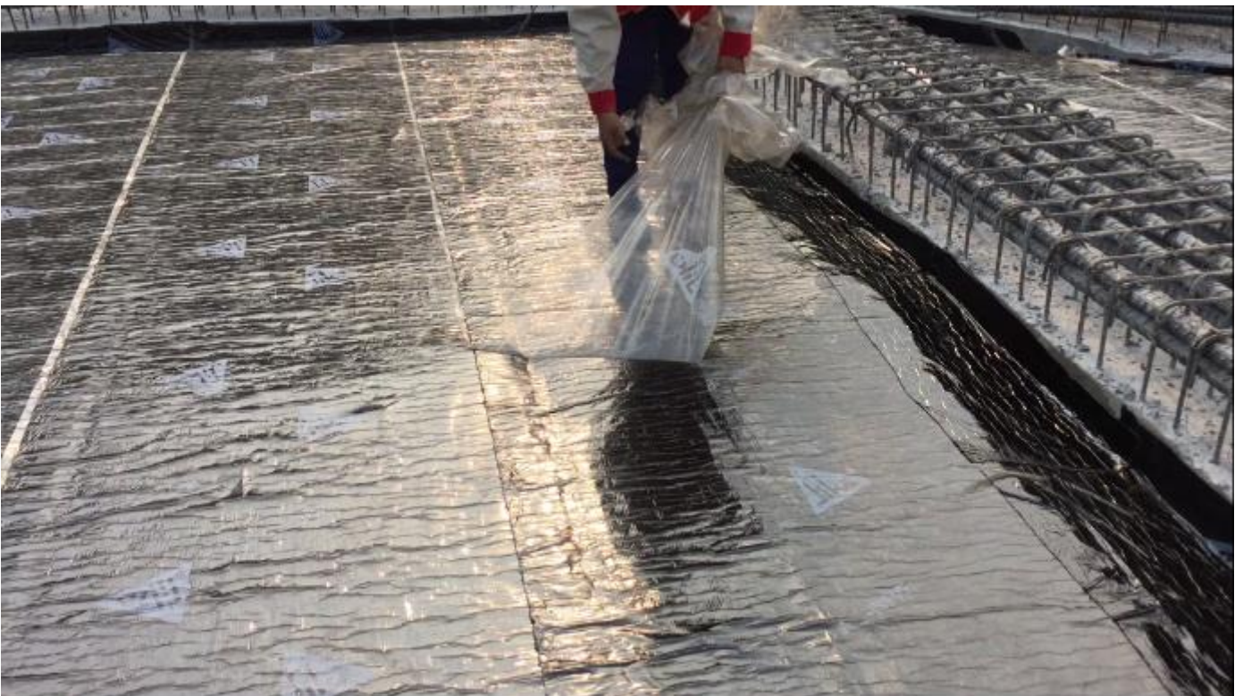
Picture: SikaBit® W-15 was used at the basement of The Nassim project.
